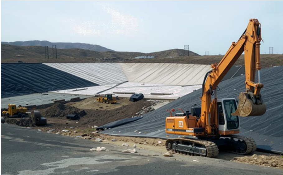
Fig. 7. Creation of an anti-filtration screen using geotextile material during the construction of a landfill for waste storage
