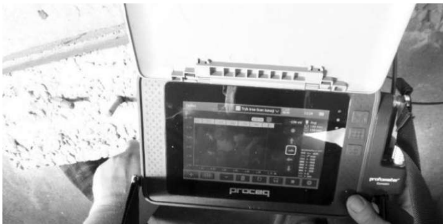
Fig. 17. Scanning in the curtain wall of a large-panel building of the diameters of: the hanger, the anchor rod and the reinforcement mesh
